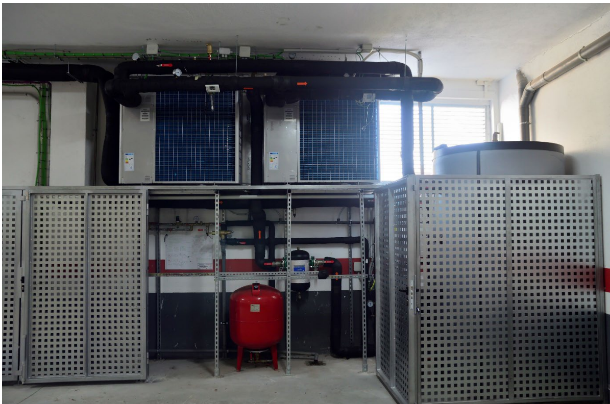
Figure 1. Central part of the installation in a demonstration site (Pasaia, Gipuzkoa, Spain)
